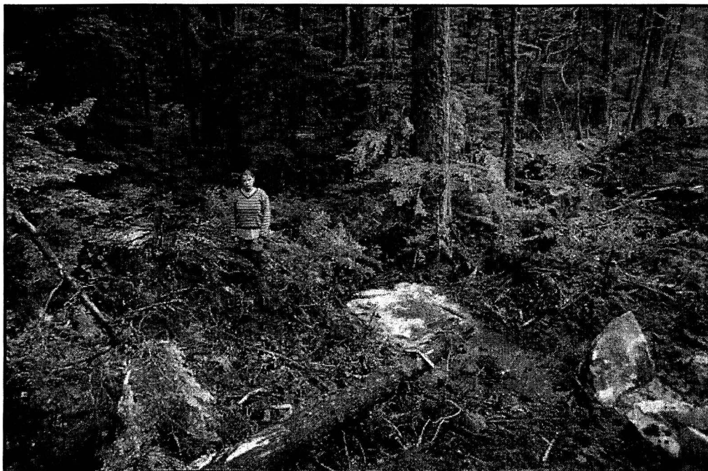
Roadbuilding in the Ingram Mooto wilderness in coastal British Columbia, July 1998. The Ingram Mooto Polallie watershed complex is the heart of the Great Bear Rainforest along BC's mid and north coast. The Ingram is home to bear, cougar, wolf, marbled murrelet, wolverine, salmon, elk, and more than 80 other birds and mammals. This pristine area is one of dozens throughout the Great Bear Rainforest slated to be clearcut by Western Forest Products (WFP) and other companies in coming years. WFP began roadbuilding in the Ingram this July. Activists from the Forest Action Network (FAN) in Bella Coola, BC, staged a virtual blockade of the road by taking pictures of the destruction with a digital camera and downloading them via satellite phone to FAN's Web site. The Western red cedar stump shown here is from a tree cut to make way for a road along Ingram Lake. The tree was roughly eight-feet wide and 900-years old.
